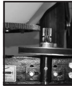
Fig.23: Gap between drive assembly and mixing drum gear.
